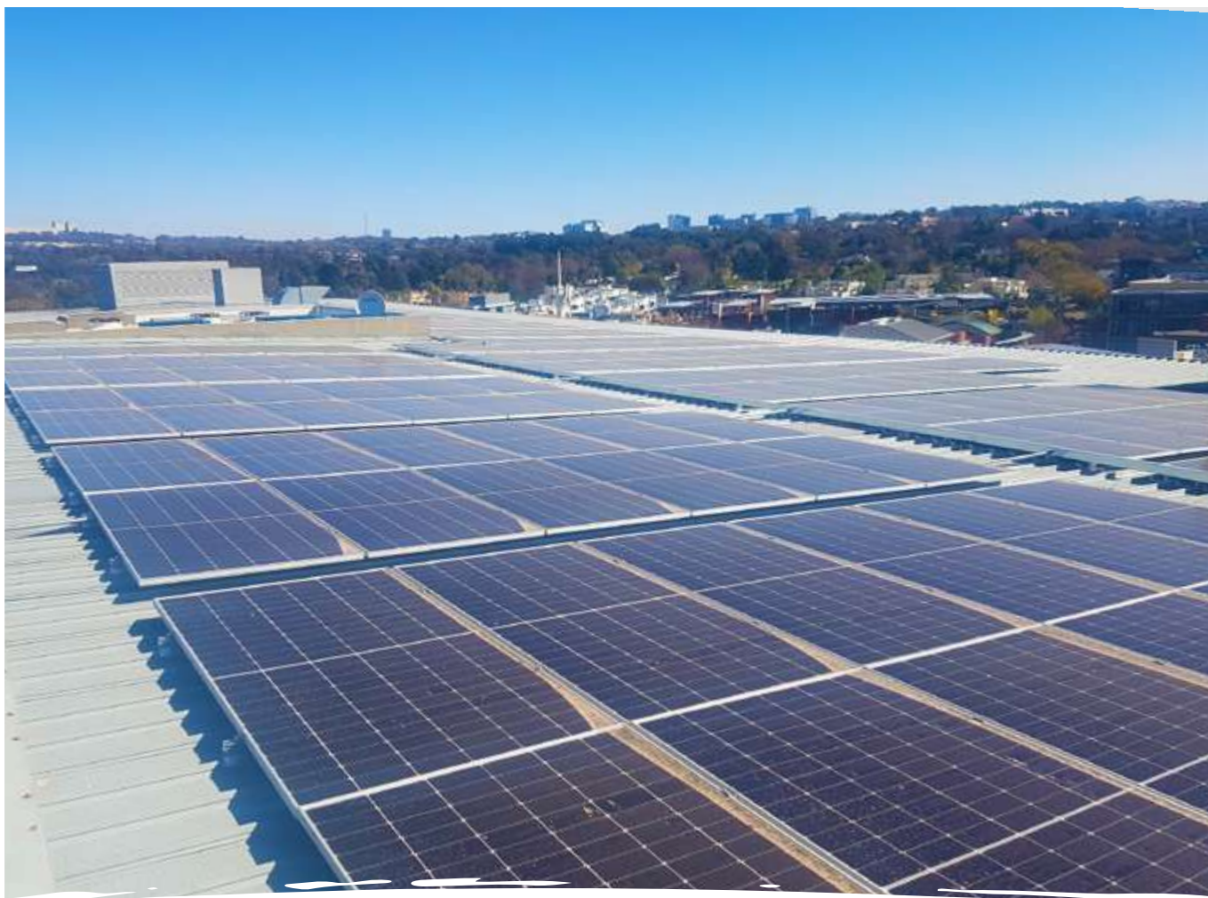
Solar panels installed on our office in Johannesburg, South Africa.
